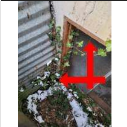
Vegetation growth in window well south side of home
