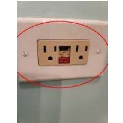
Inoperable electrical receptacle in second floor hallway bathroom
