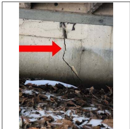
Vertical crack of exterior concrete stem wall from the basement south side of home
