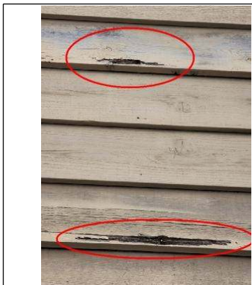
Damaged exterior wood siding South West exposure
