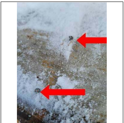
Protruding fasteners of tread at steps to decking
