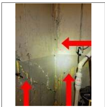
Patched vertical cracks of foundation stem wall North east side of basement
