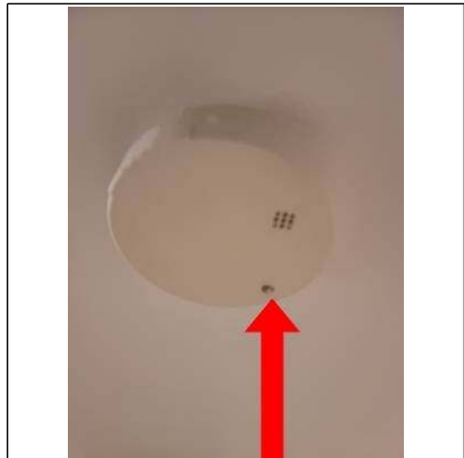
Inoperable smoke detector in basement
