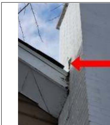
Detached aluminum flashing of chimney Chase east side of home
