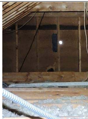
Hole in exterior wall of east side of attic
