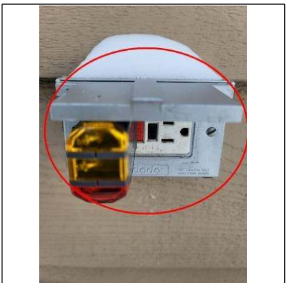
Inoperable exterior electrical receptacle east side of home
