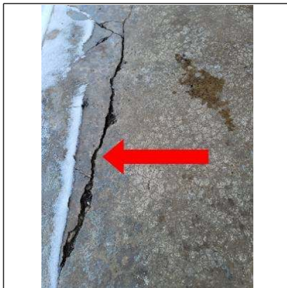
Cracked concrete of garage floor
