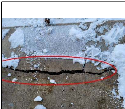
Cracked concrete of garage floor
