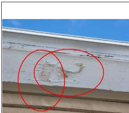
Peeling paint of wood soffit material south side of roof
