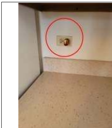
Non GFCI electrical receptacle above kitchen countertop
