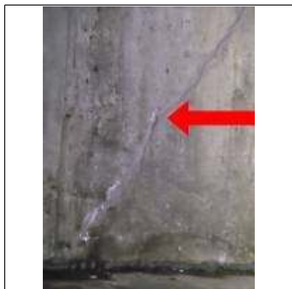
Vertical crack of foundation stem wall South side of crawlspace
