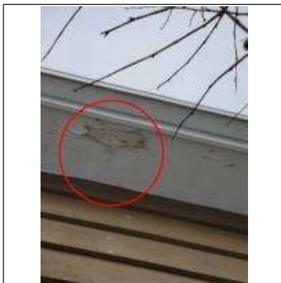
Peeling paint of wood soffit materials south side of roof
