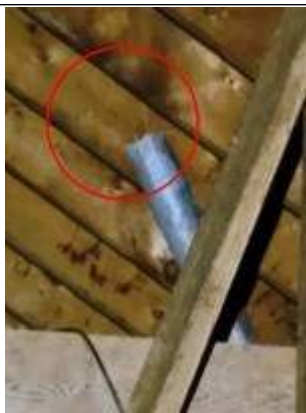
Bathroom vent fan exhausting into the Attic
