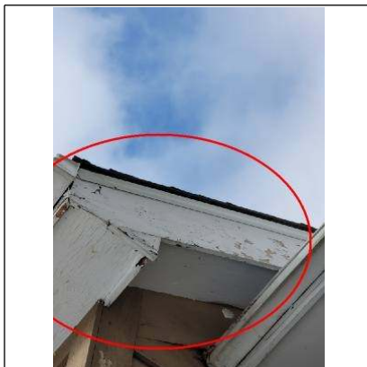
Deteriorated and peeling paint of wood fascia and soffit materials
