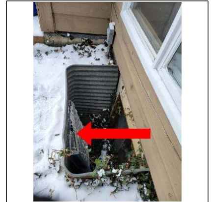
Improper installation of window wall cover
