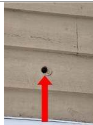
Hole in exterior wood siding east side of home
