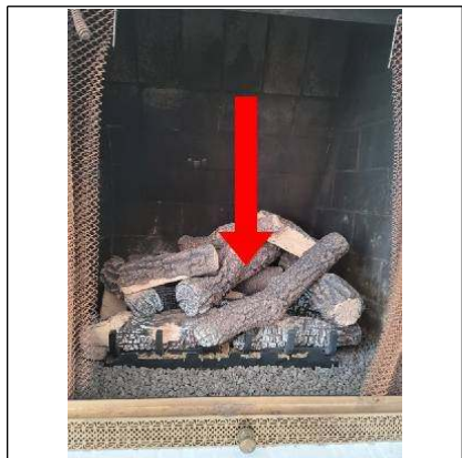
Inoperable gas fireplace appliance
