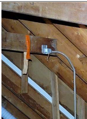
Open electrical junction box in the Attic
