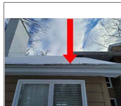
Damaged and detached gutter first floor North exposure
