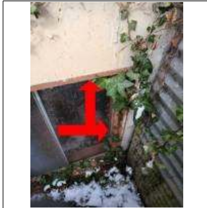
Rusted window well frame south side of basement
