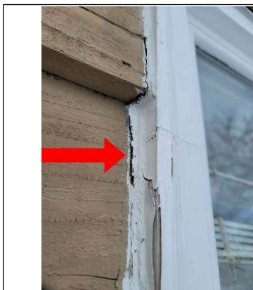
Dried and cracked exterior caulking of window penetration south side of home
