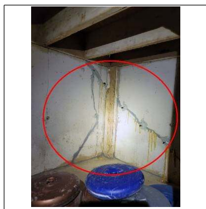
Patched Vertical cracks in foundation stem wall north side of basement
