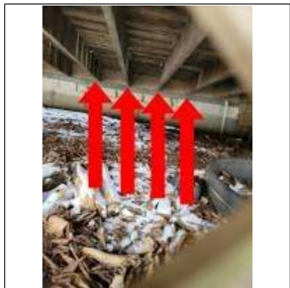
Missing joist hangers of decking south side of home
