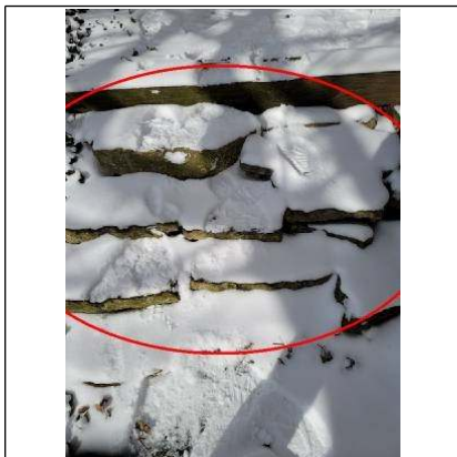
Improper configuration of steps at elevation change at the Southwest area of the grounds
