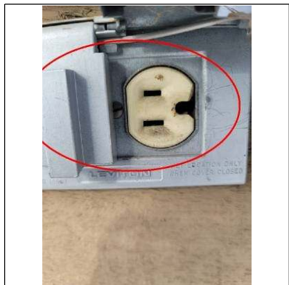
Non GFCI exterior electrical receptacle south side of home
