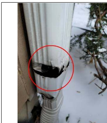
Damaged and detached downspout connection Southeast corner of home
