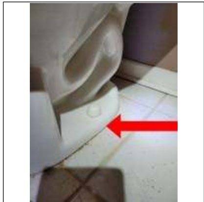
Loose toilet bowl second floor primary bathroom
