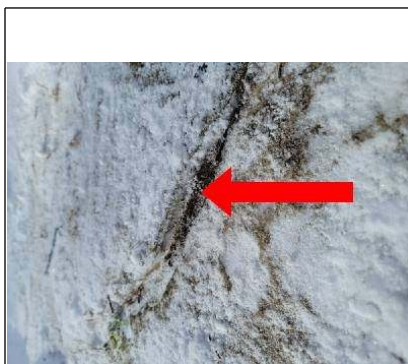
Cracked and settled concrete service walk south side of home
