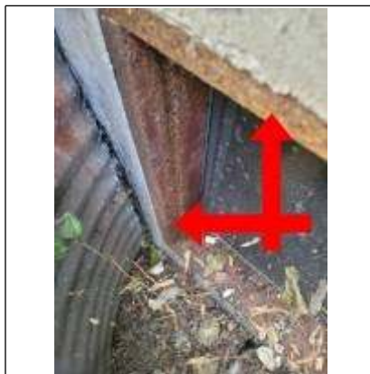
Rusted window well frame east side of basement
