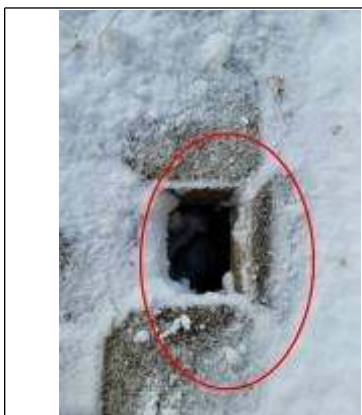
Missing drain cover of service walk at South entrance to garage
