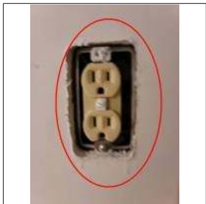
Missing protective cover plate of electrical junction box in basement
