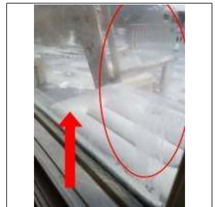
Evidence of failed thermal insulation seal of ground level window south side of home
