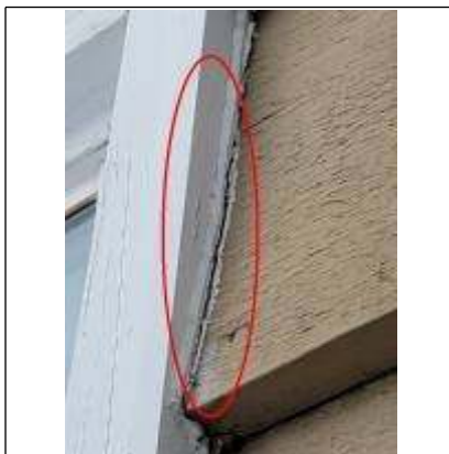
Tried and detached sealant of exterior window penetration south side of home
