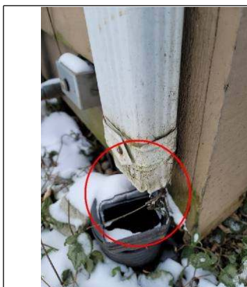
Detached downspout from extension northeast corner
