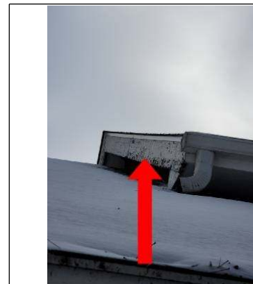
Peeling paint of exterior wood fascia materials yeast exposure over living room
