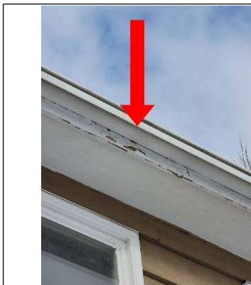
Deteriorated and peeling paint of wood fascia materials south side of roof
